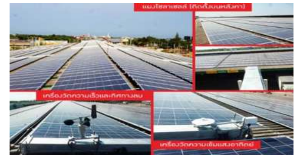
SGG Solar roof 0.988 MW
